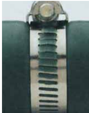
HOSE INSTALLED WITH UNLINED CLAMP
